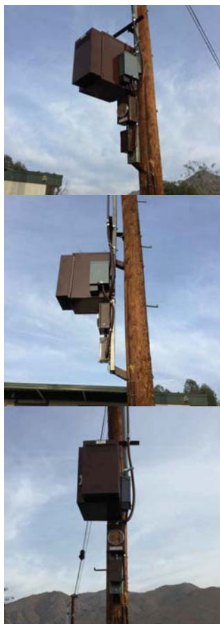
EQUIPMENT ON POLE:
