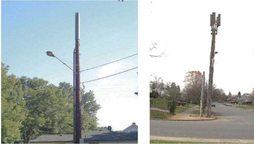
Figure 15-6 Pole Top Antenna Attachments
